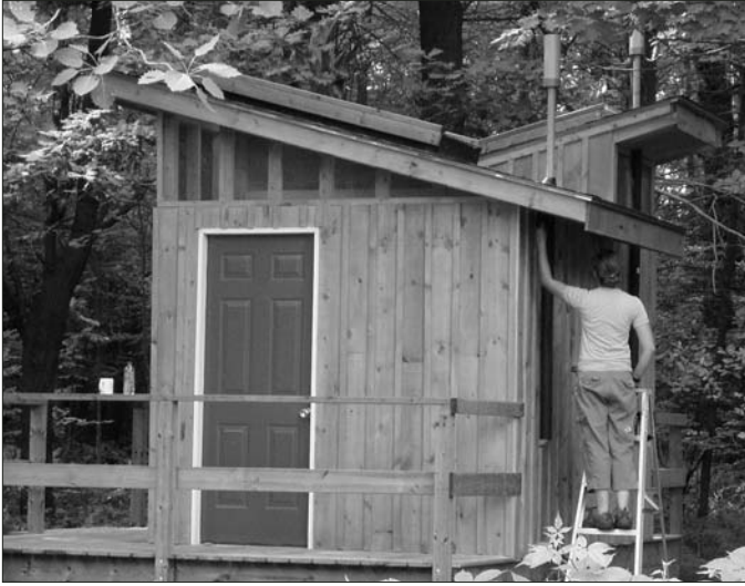
Summer student Jacqui Kerr puts finishing touches on a new washroom building at Grant's Woods. The building features environmentally-friendly composting toilets, and is designed for use by student groups and other visitors to the trail system.
